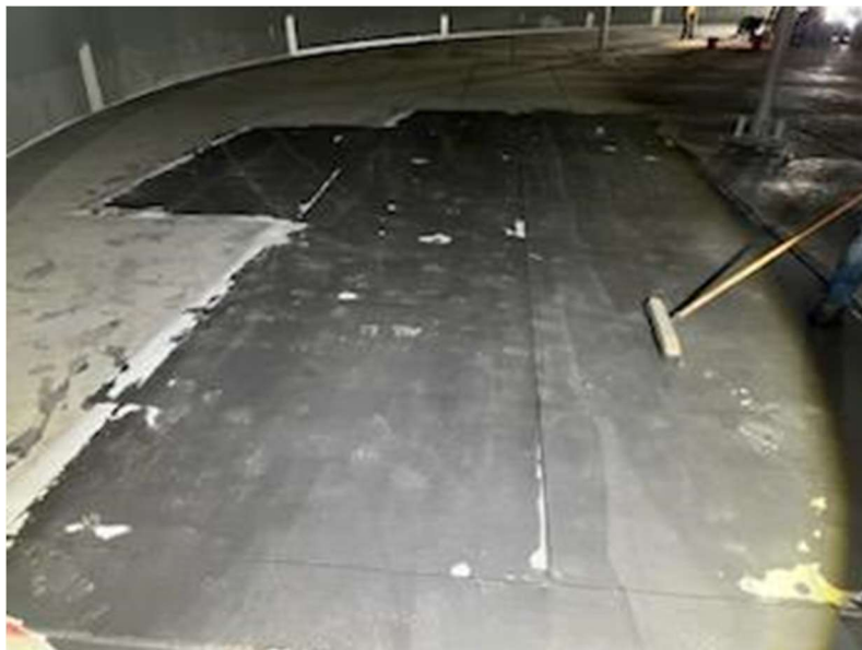
View of heavy paint layer and mil scale requiring a more aggressive blasting technique to speed up removal.
