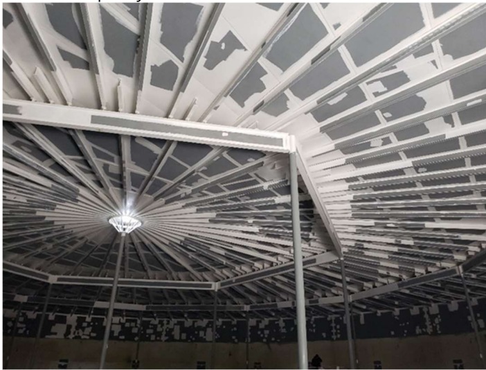
View of ceiling epoxy stripe coating which is complete and ready for final spray coating.
