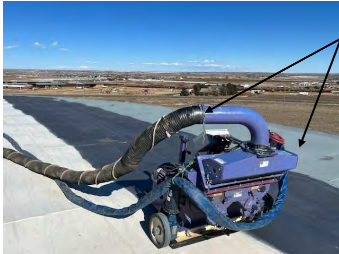
Roof sandblasting with robotic blaster followed by zinc priming in preparation for exterior top coat.
