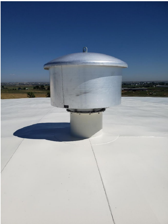
New roof vent installed and functions significantly better than the original vent.
